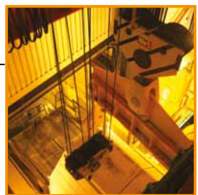
CASK HANDLING CRANE
